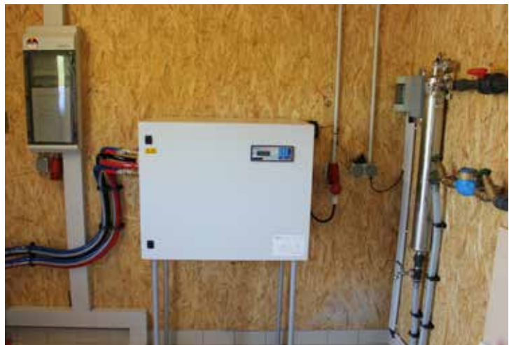
Power distribution board, switch cabinet, UV module
